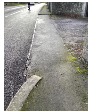
Figure 4.5: Inappropriate vehicle crossover
