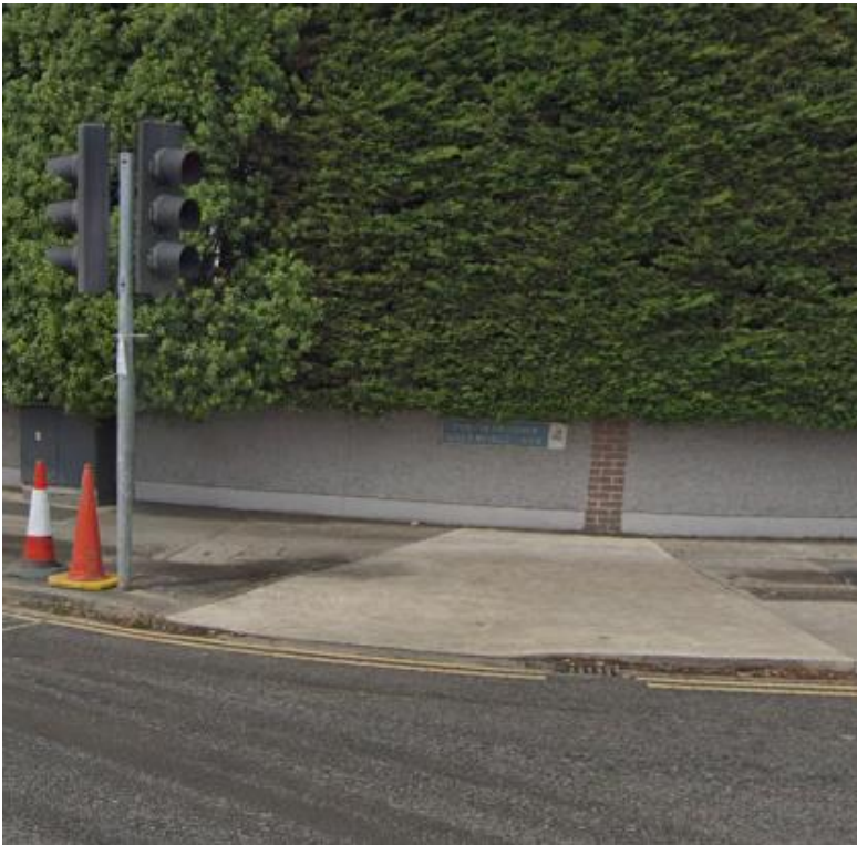
Figure 2.7: Missing tactile paving
