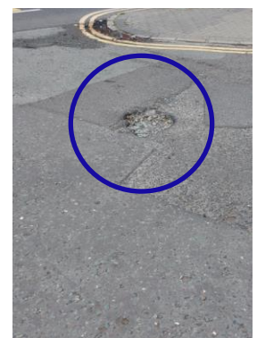
Figure 3.9 Pothole at Junction Bellmouth
