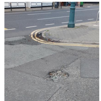
Figure 2.6 Evidence of ponding in the carriageway at Eglinton Terrace/ Donnybrook Rd junction
