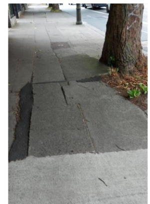
Figure 2.5 Trip Hazards along Leeson Street Upper due to impact of roots on mature trees
