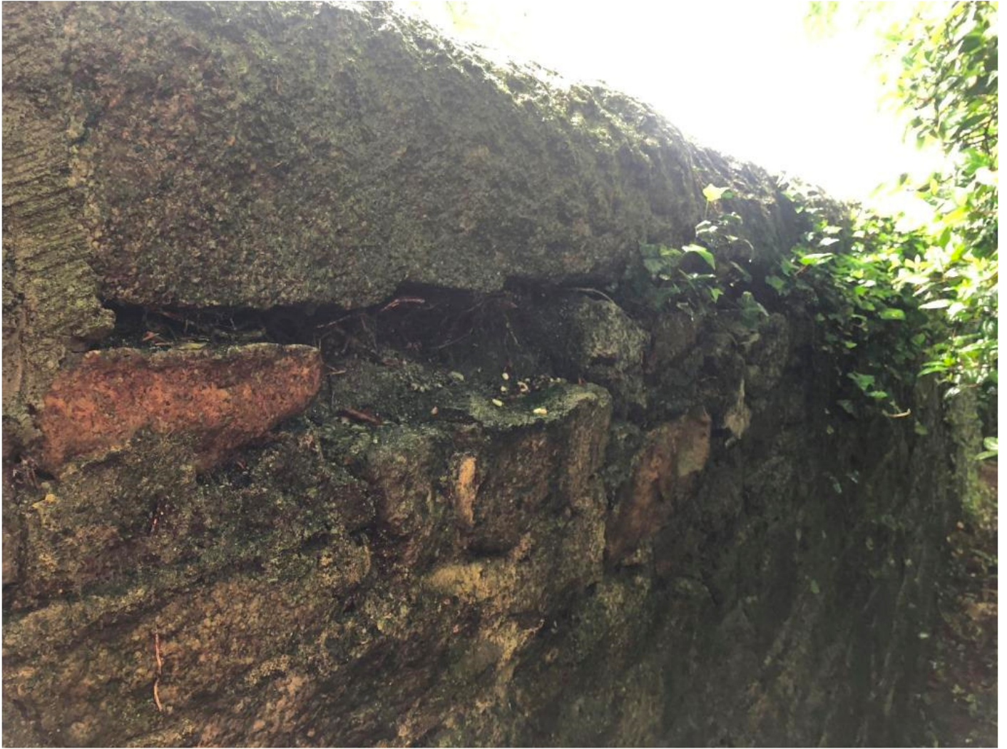
Figure 11, Missing blockwork noted at top of east wall
