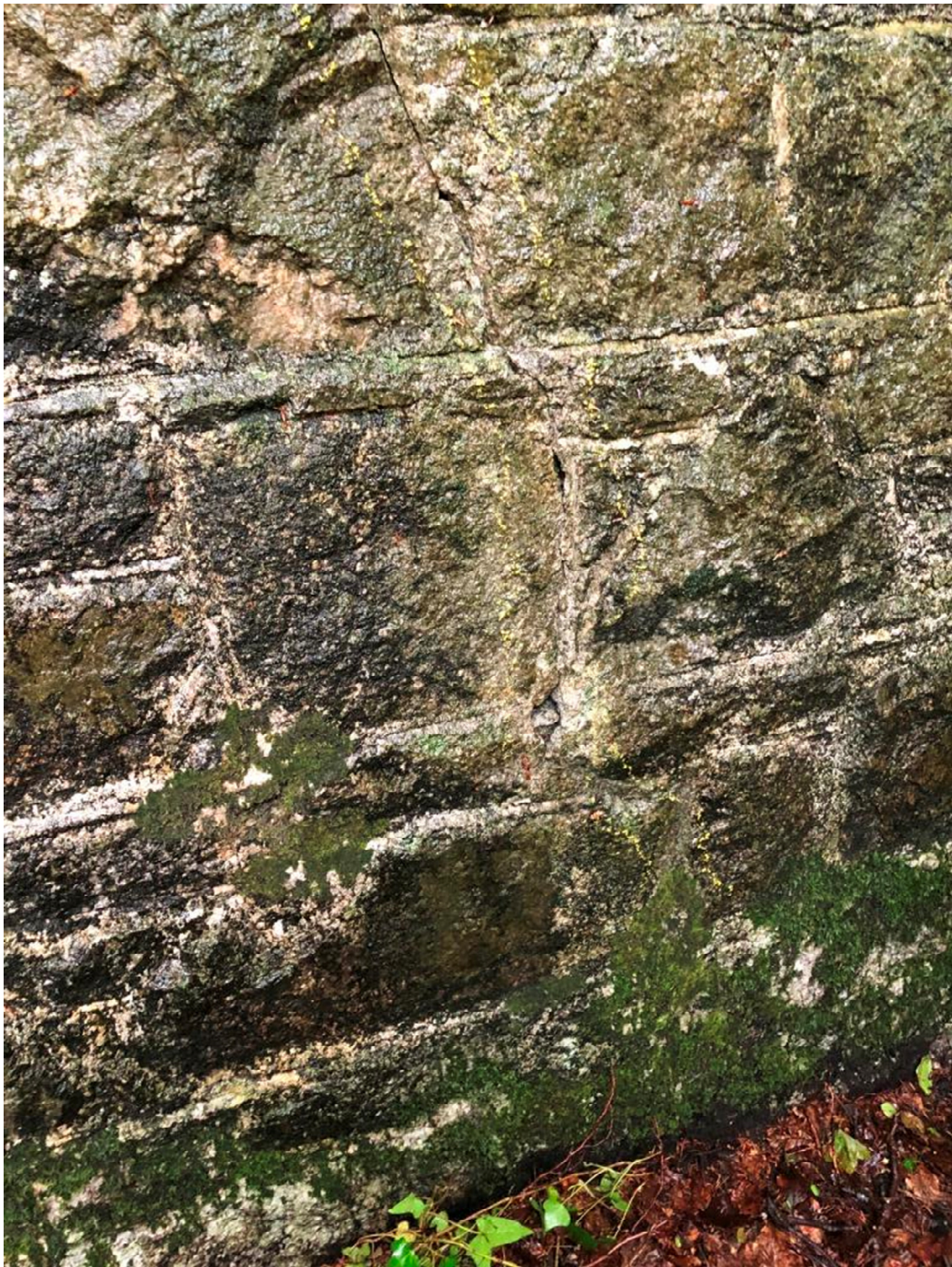
Figure 10 Vertical crack noted on east elevation
