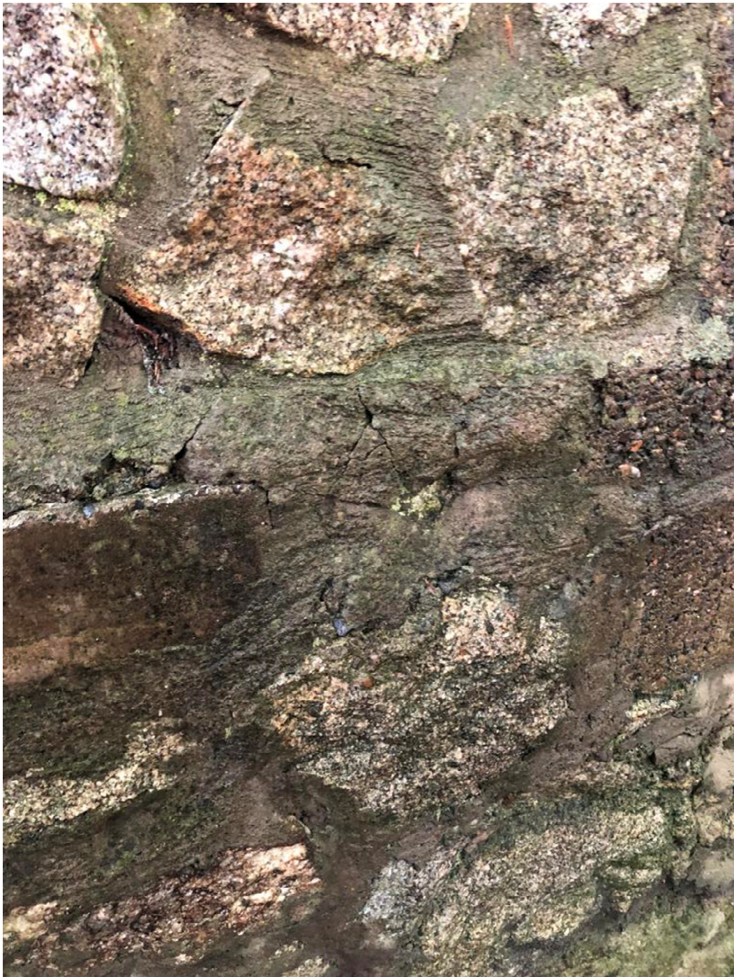
Figure 12 Hairline cracks noted at multiple locations
