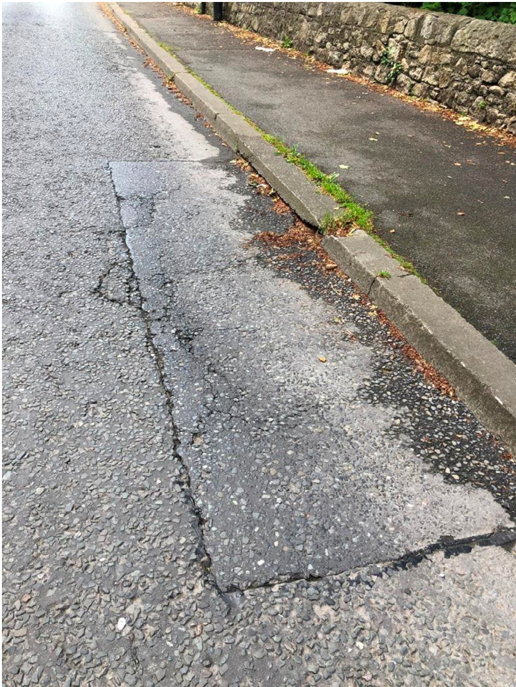
Figure 21 Damage to west kerb and carriageway noted
