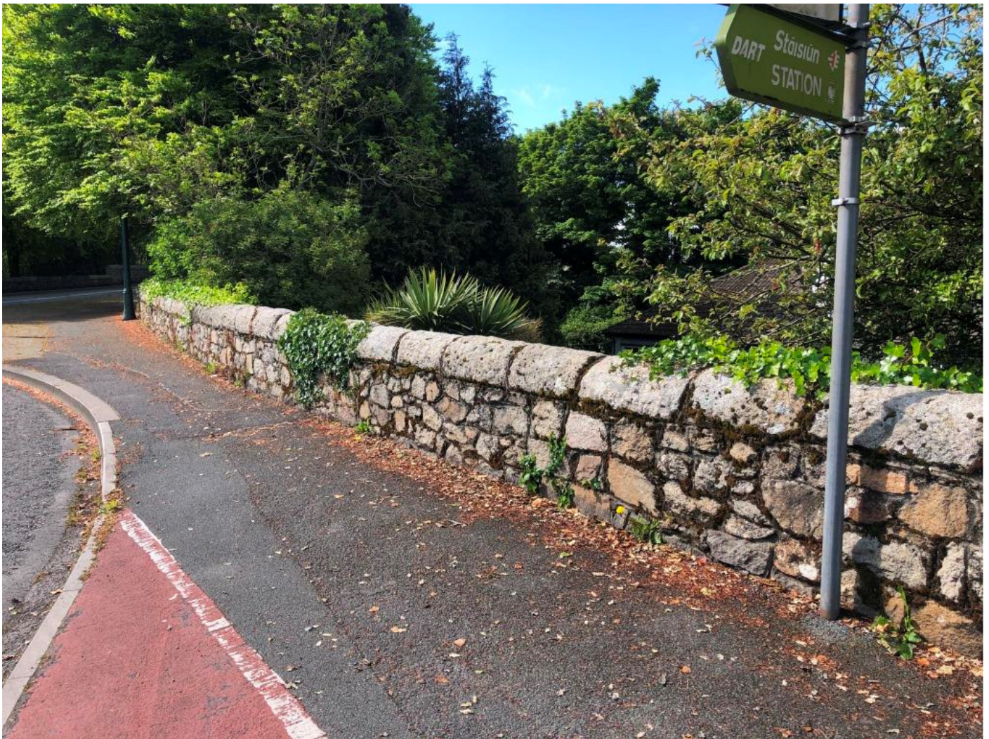
Figure 18 Areas of mortar loss and algae growth on the west parapet. General wear noted on footway surfacing
