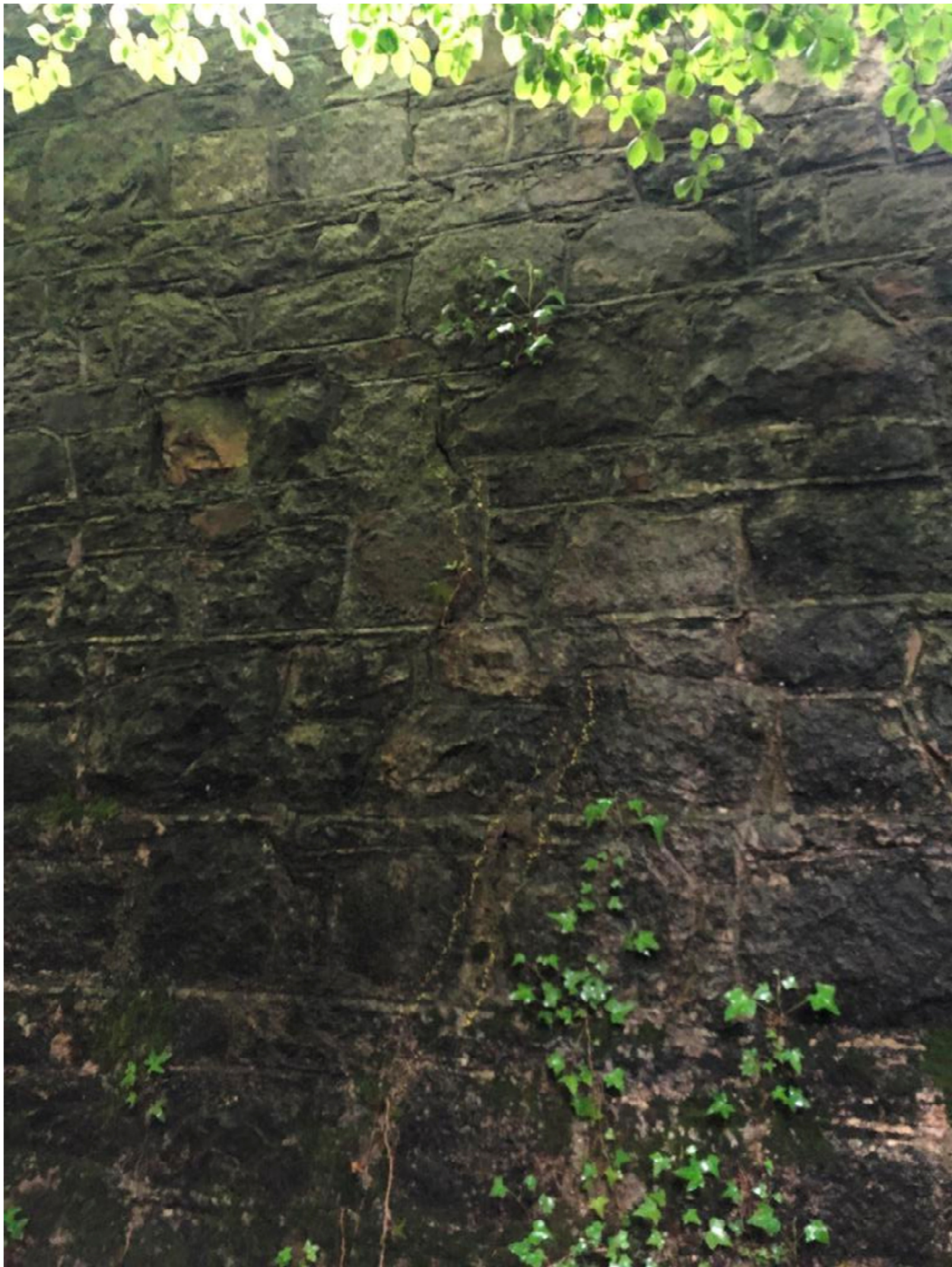
Figure 8 Vertical crack noted on east elevation
