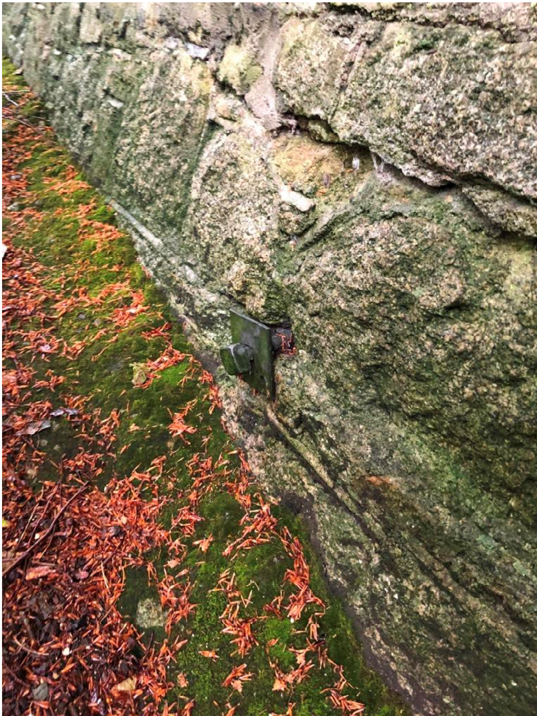
Figure 13 Exposed tie bar noted on east elevation
