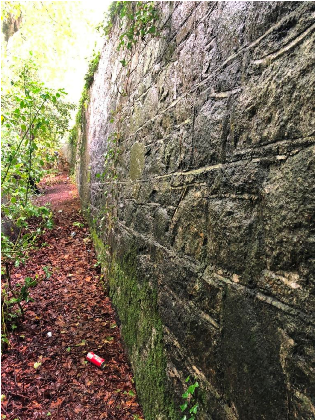
Figure 9 Algae growth noted at base of east wall.
