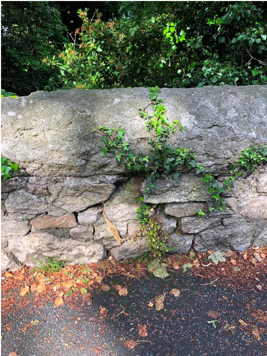
Figure 19 Missing blockwork noted on south west parapet
