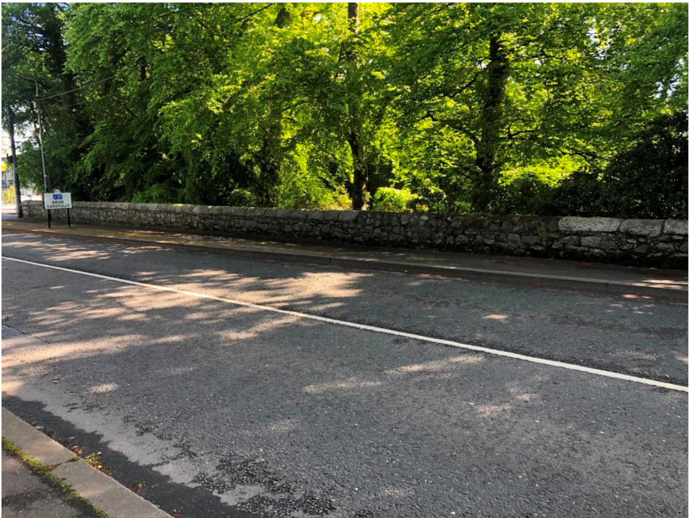
Figure 20 East parapet in generally good condition. Areas of mortar loss and Algae growth noted.
